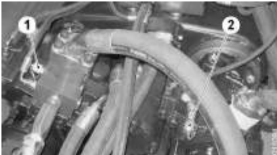
Measuring outlet, hydraulic oil pumps
