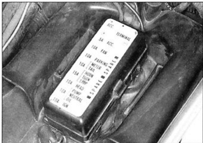
5.1a The accessory fuses are beneath a cover inside the top compartment . . .
