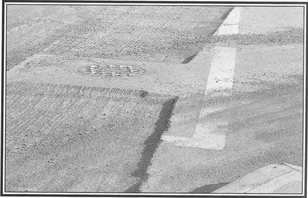
These steep edges are a big hazard to motorcyclists.
