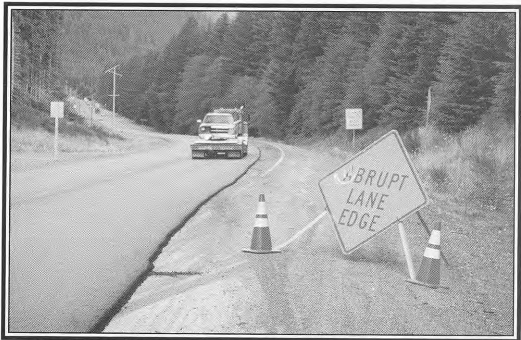
Heads up! That pavement edge ahead wanders across your lane.
