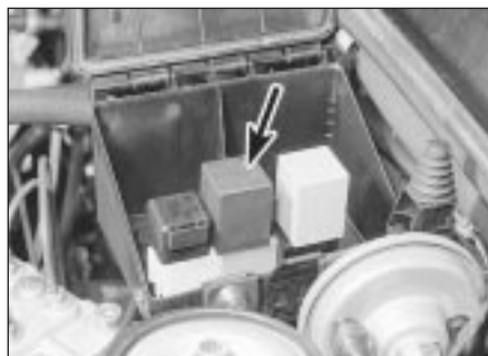
23.9 ABS surge arrester relay (arrowed)
