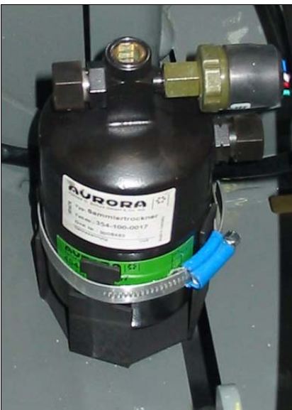
Fig. 1: Dehumidifier with pressure switch
