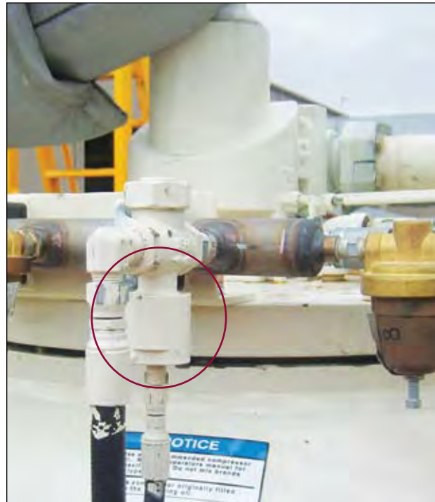
System (Shutdown) Blowdown valve
