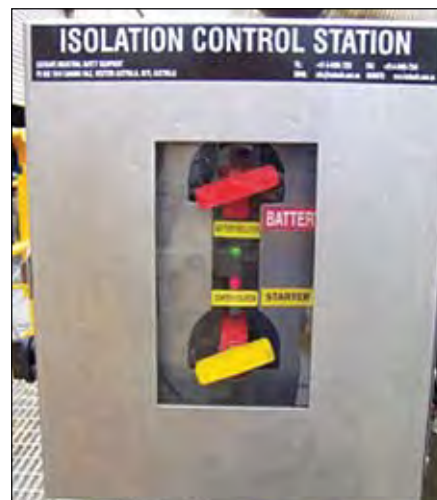
Battery Isolation Station
