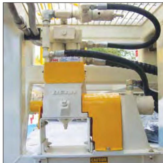
Water Injection Pump
