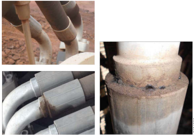
Fig. 224: Moist surfaces, no visible oil leak
