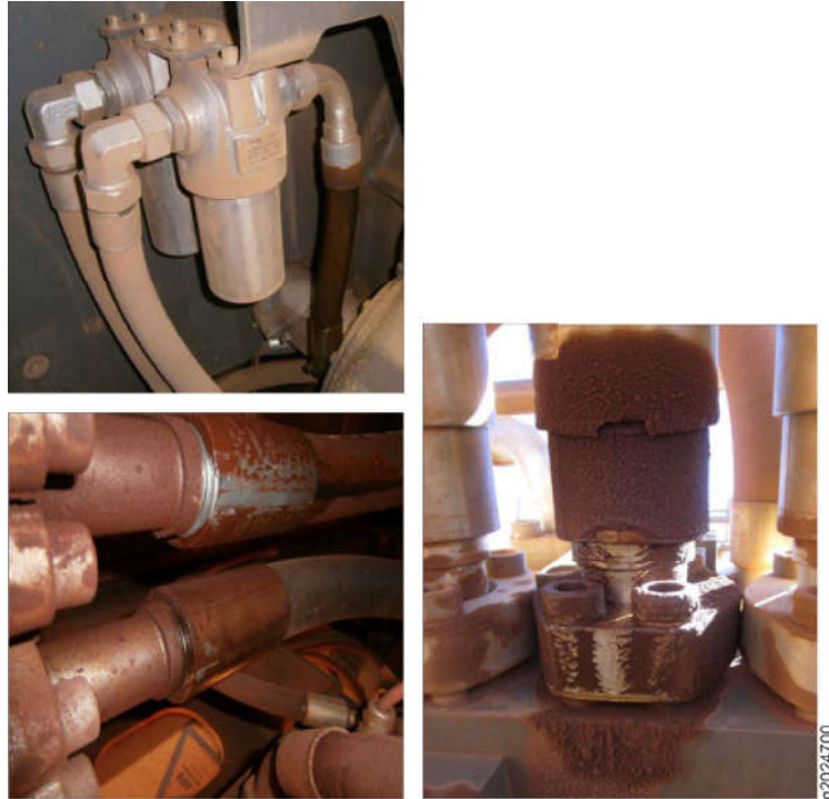
Fig. 249: Moist surfaces, slight oil leak visible
