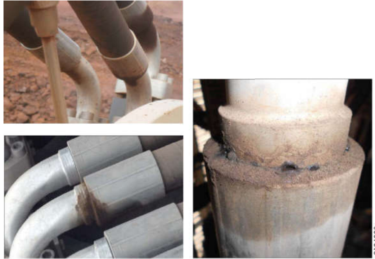
Fig. 247: Moist surfaces, no visible oil leak
