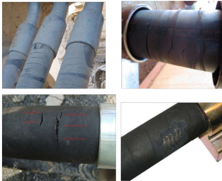
Fig. 245: Cracks or cuts up to the steel fabric or steel fabric exposed due to damage to the outer jacket
