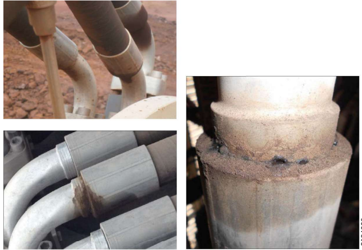
Fig. 242: Moist surfaces, no visible oil leak
