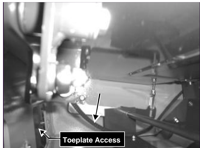
Fig. 6-66 The auxiliary cable routing underneath the floor plate.
