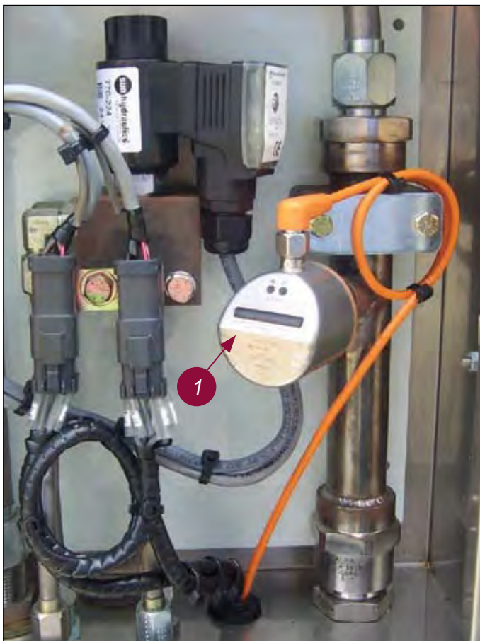
Water Injection Flow (Transducer Cabinet)
