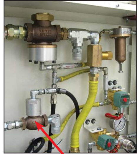
Fig. 4-24 System Blowdown Valve
