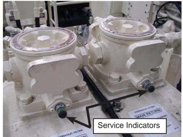
Fig. 9-11 Return Filters Mounted on Hydraulic Tank
