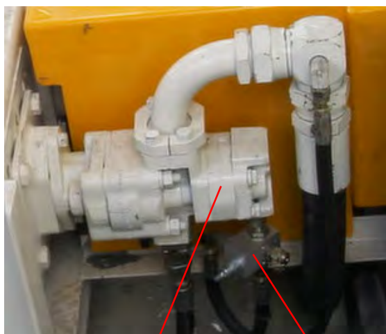
Air Conditioner Pump and circuit Relief Valve
