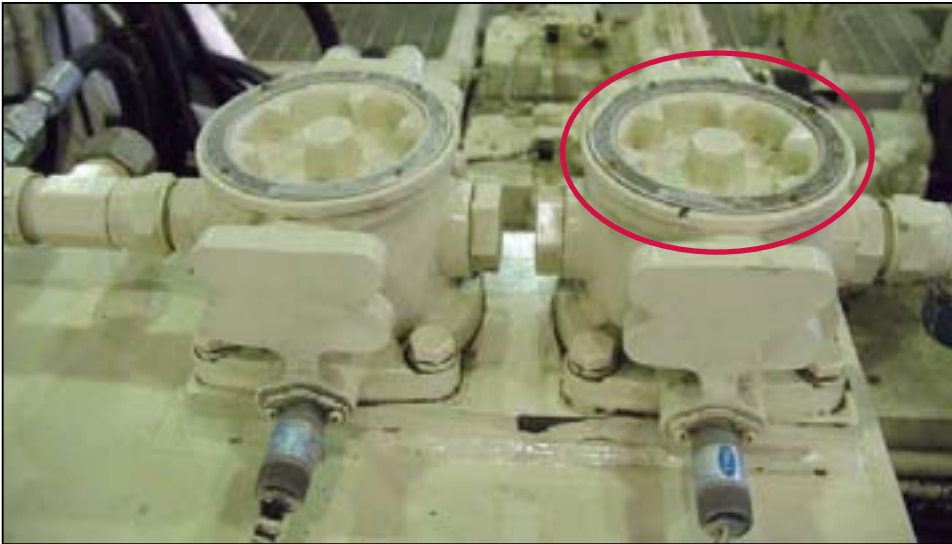
Return system flow is filtered at the reservoir
