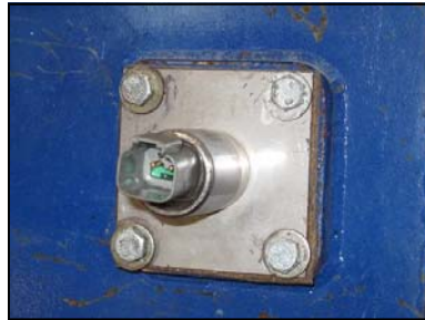
Engine Coolant Level Sensor
