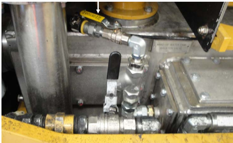
Main Supply/Isolation Valve
