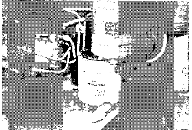
Install new primary and final fuel filters.
