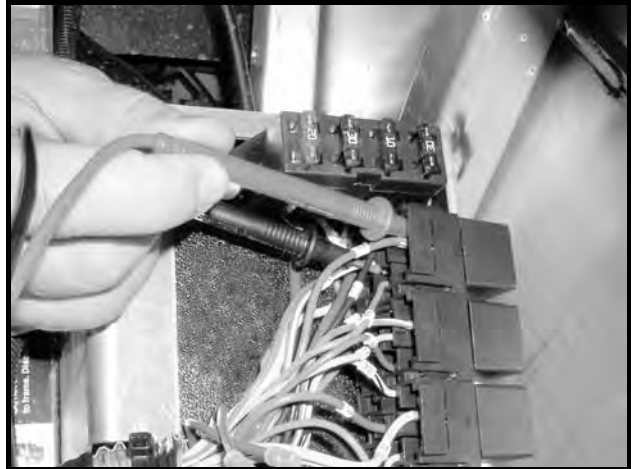
Figure 11c-16 Start Relay Contact Test
