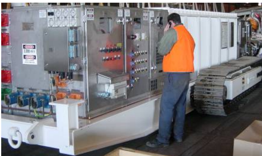
Transformer station and crawler unit
