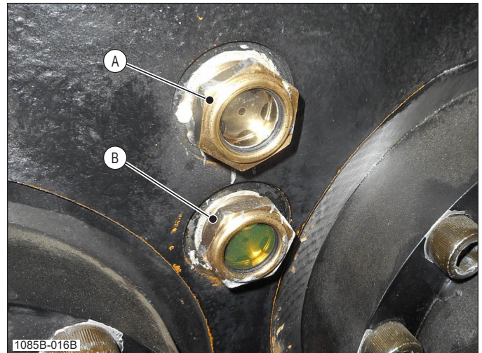
Crane Slew Oil Level (Ealier Design)
