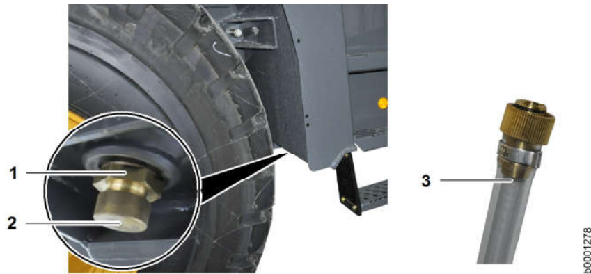
Fig. 333: Draining off condensate and sediment from the fuel tank
