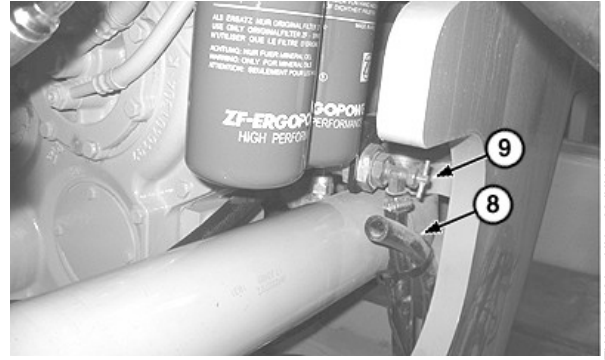
Hydraulic Oil Drain Valve and Hose
