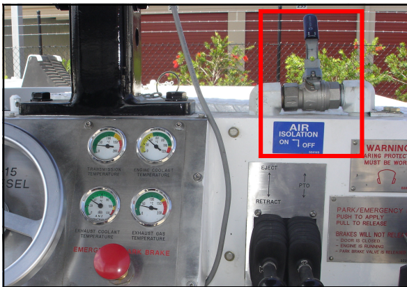
Figure 5.2.1 - Main Air Isolating Valve
