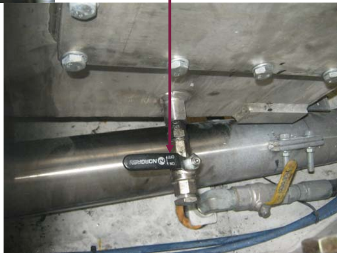
Low Water Shutdown Test Ball Valve
