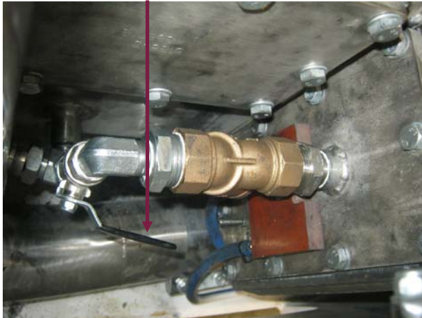
Main Supply/Isolation Valve
