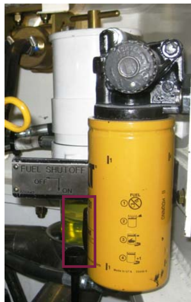
EMERGENCY FUEL SHUT OFF VALVE
