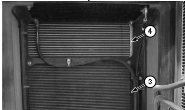
Hydraulic Oil Cooler and Radiator
