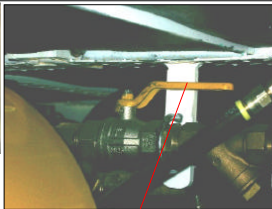
Figure 4.1.2 Main Air Isolating Valve
