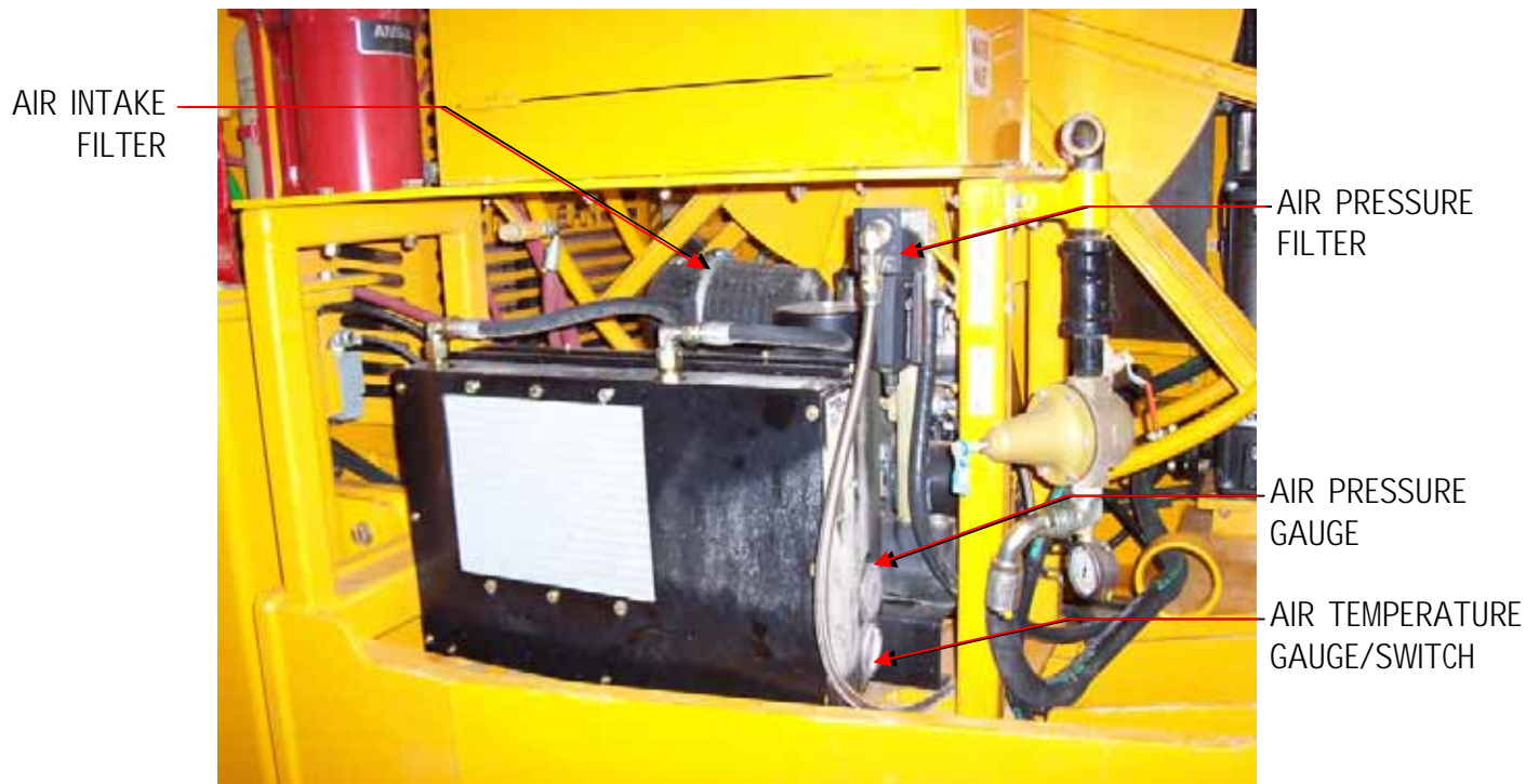
Figure 11 – Air Compressor Located in Rear Deck Assembly
