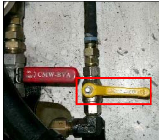
Figure 6.10 - Air Receiver Drain Valve
