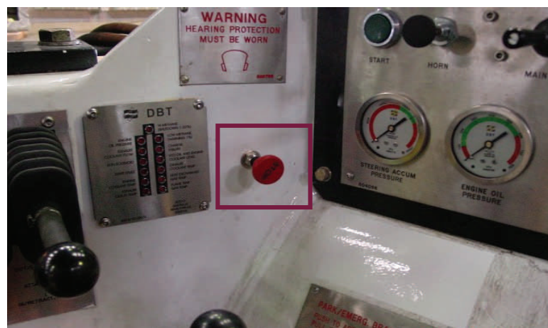
EMERGENCY INTAKE SHUT OFF VALVE ACTIVATION BUTTON
