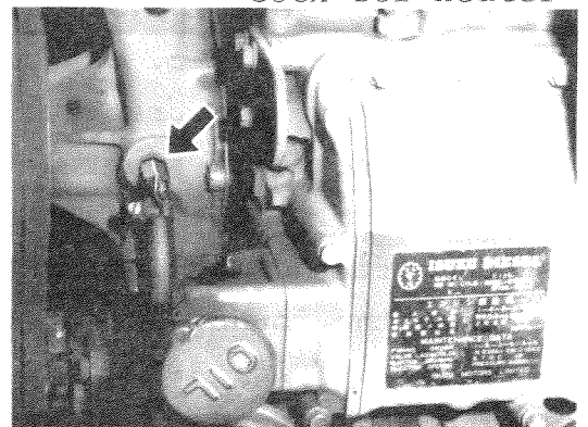
Photograph 3-4 Hot Water Inlet Cock for Heater
