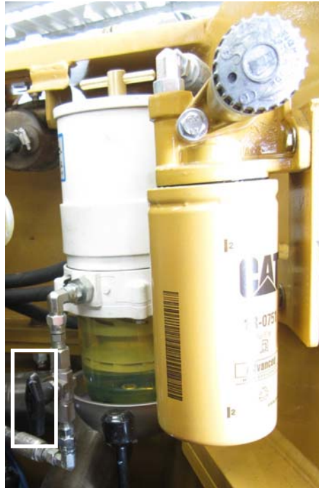
EMERGENCY FUEL SHUT OFF VALVE
