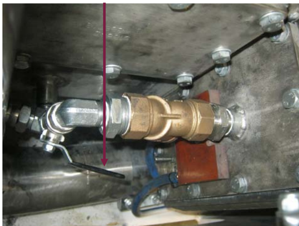
Main Supply/Isolation Valve
