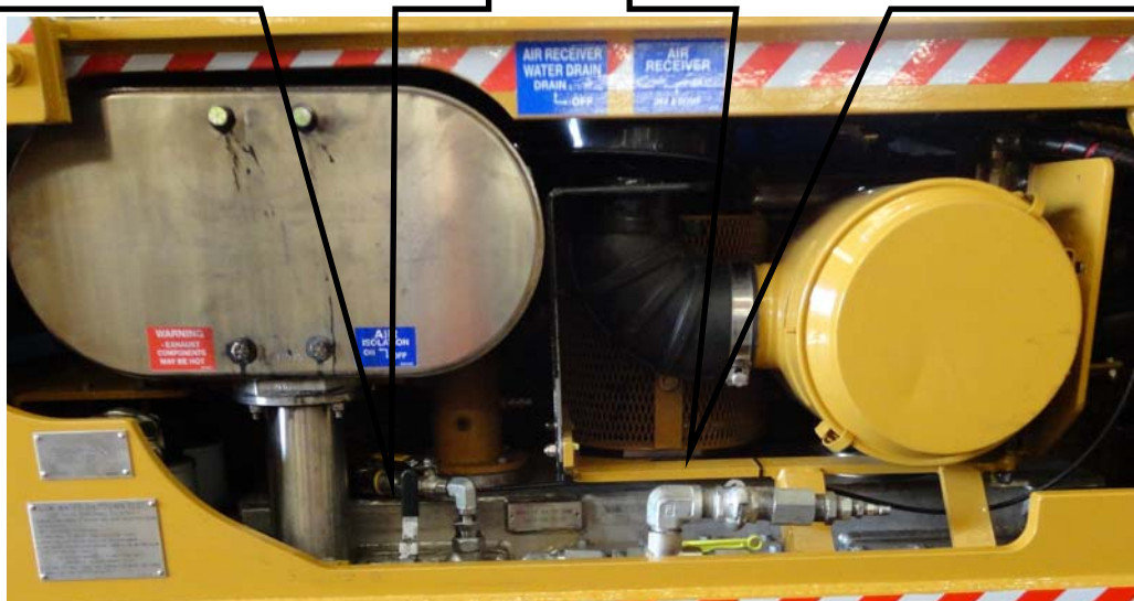
MAIN AIR MANIFOLD
