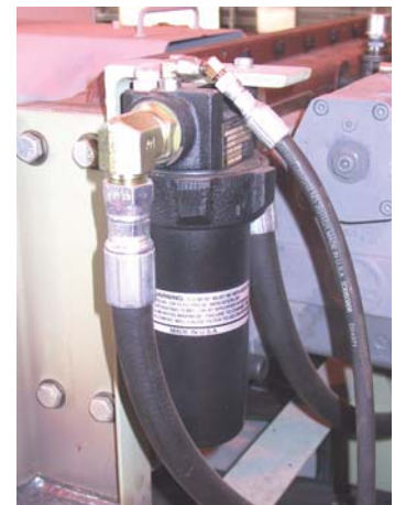
Fig. 4-10 Hydraulic Pump Charge Filter—One filter mounted on each side of pump drive.
