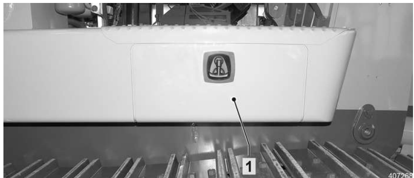
Access – refueling pump
