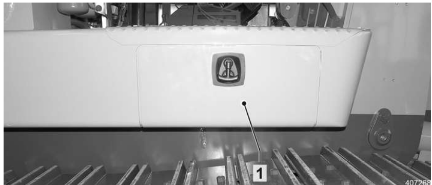
Access – refueling pump
