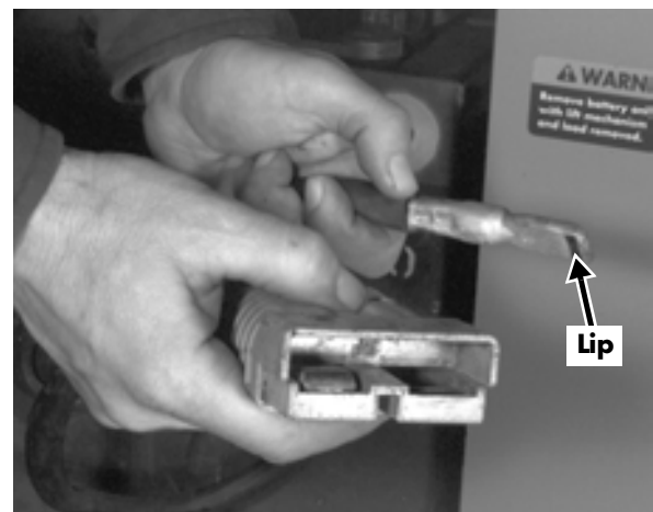
Figure 5-22: Cable Removed from the Battery Connector
