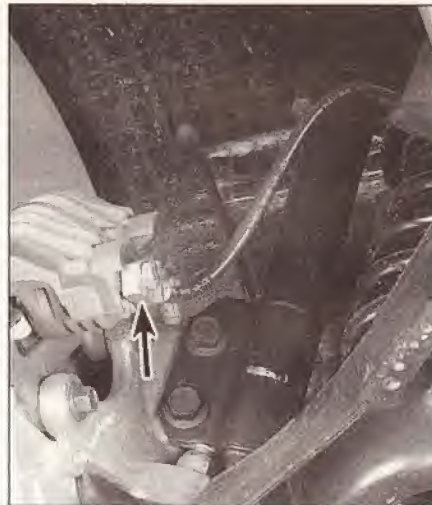
18.11 Check along the brake hoses and at each fitting (arrow) for deterioration and cracks
