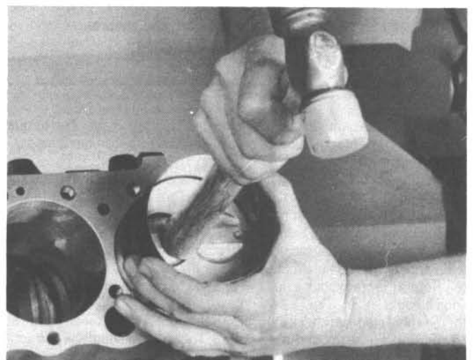
24.11 Drive the piston gently into the cylinder bore with the end of a wooden or plastic hammer handle
